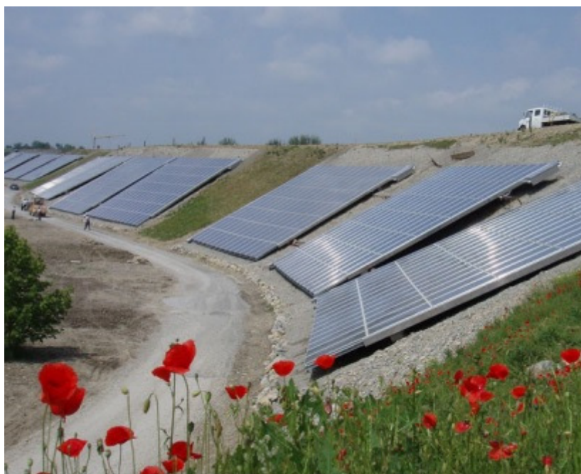
Figur 2: On a slope (Schüco), Crailsheim, Germany (by Stadtwerke Crailsheim GMBH). [1], Fact sheet 2.2
