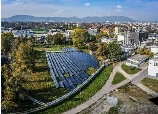
Fig. 1: Fernheizwerk Graz solar plant, part of Austria's biggest solar district heating plant
