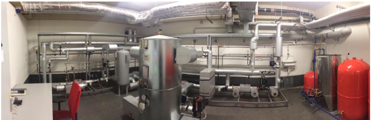
Fig. 4: Feed-in substation of the experimental plant (deformed panoramic view) [AGFW 2018]
