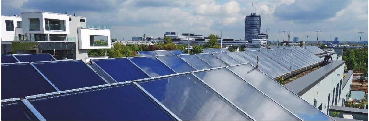
Fig. 3: Solar collector field of the experimental plant
