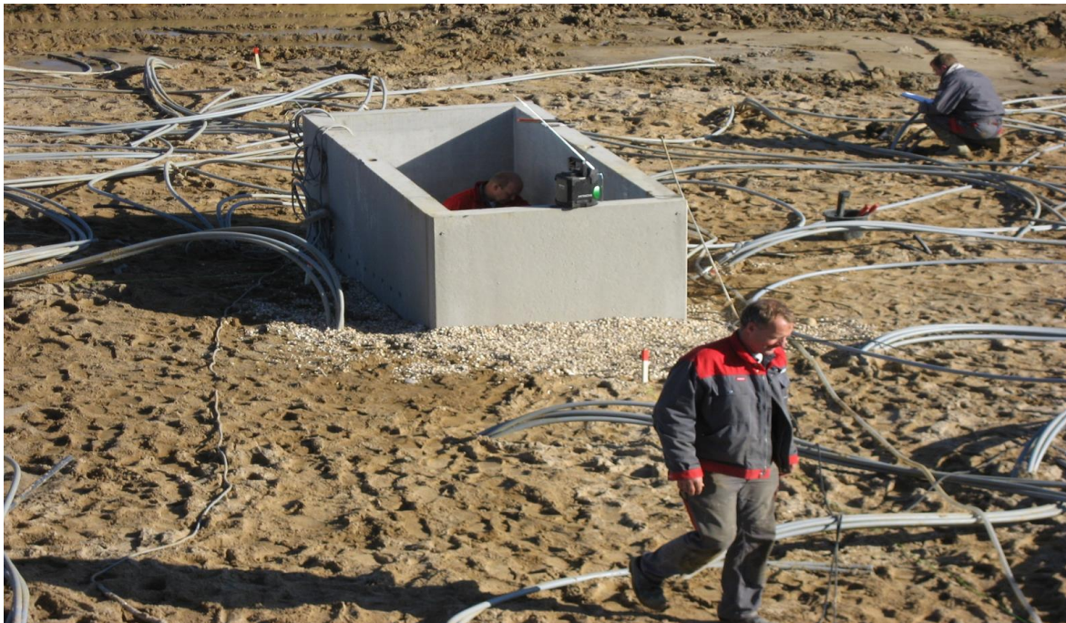
Fig. 12. Connection pipes and well. Source: PlanEnergi
