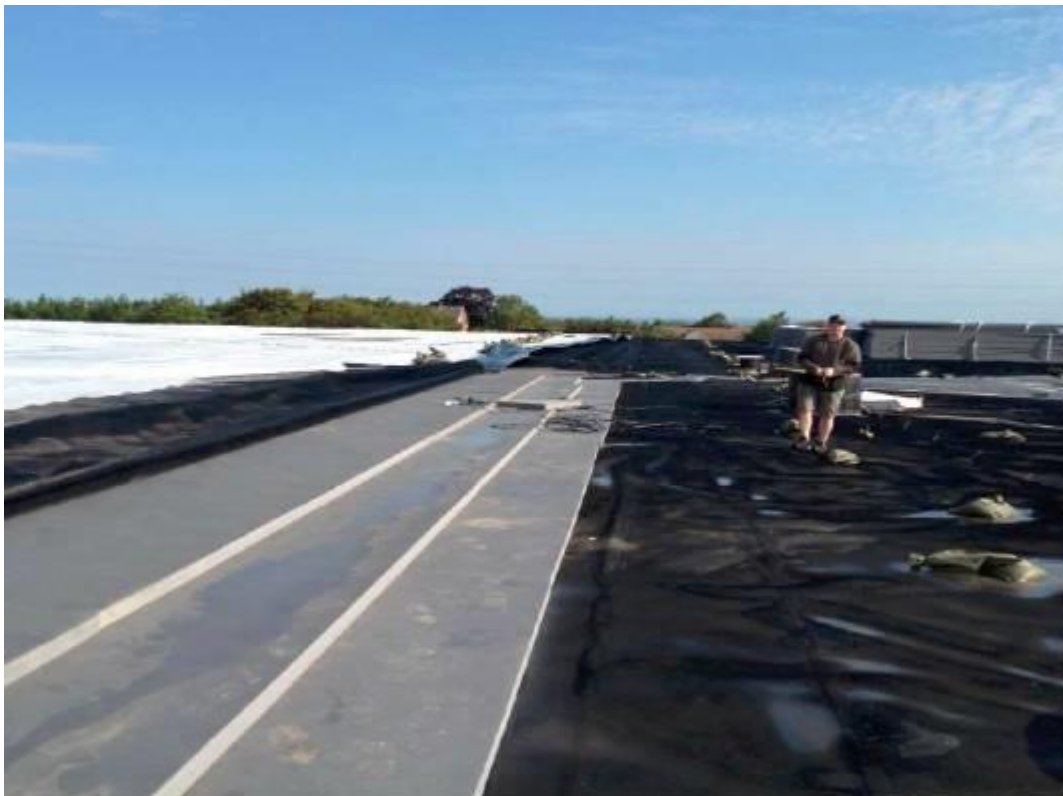
Fig. 18. Implementation of the lid, Marstal. The HDPE-liner is welded onshore and drawn on the water. Then hypernet, 3 layers of insulation and toplineer is implemented. Source: PlanEnergi
